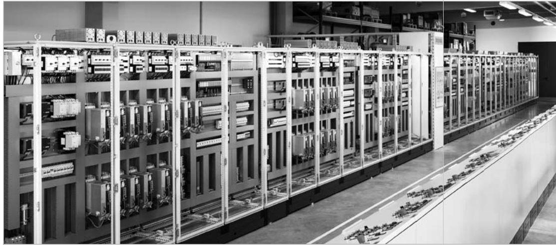
[ Part of the control room for the pipe plant in Malaysia ]
